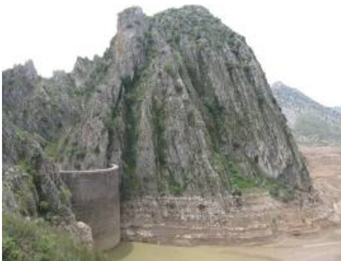
Fig. 12 Empty reservoir of Montejaque dam on Gaduares River in karst of southern Spain. Due to high leakage the reservoir was abandoned in the 1950s (photo Z.Stevanović)
